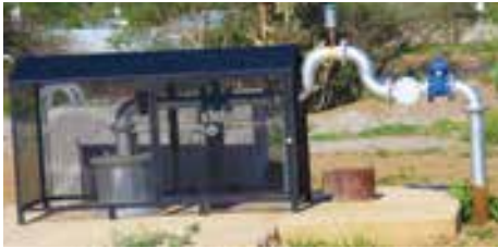
One of the new boreholes supplying about 120 m 3 of water to the city's water supply network.
